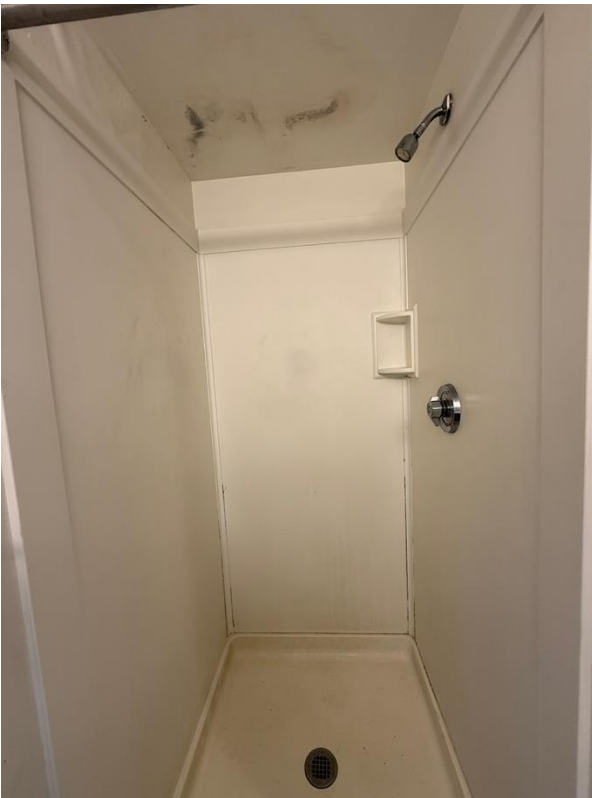
Mold Growth on Shower Ceiling
