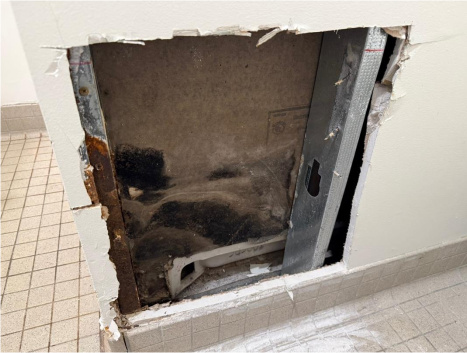
Mold Growth on Bathroom Wall
