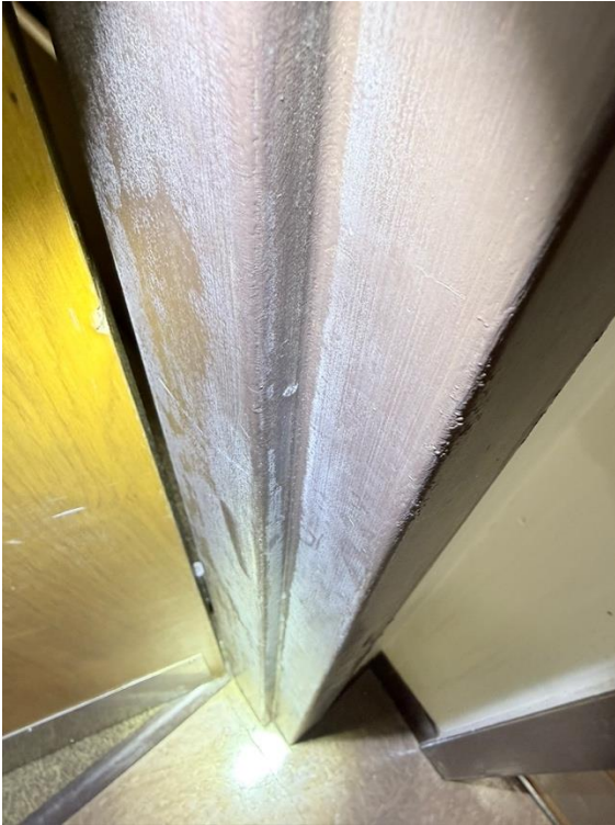
Mold Growth on Door Jamb, Located in Foyer
